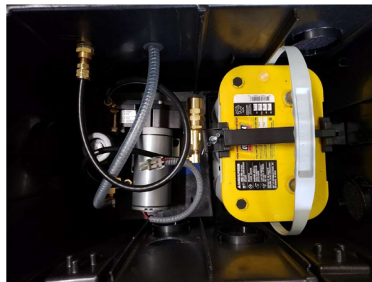
Battery installed with J-bolts
